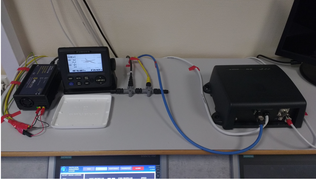
Figure IV.3: GPS receiver (left), NMEA 2000 bus (center) and AIS receiver (right) (source: personal work).
